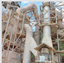
Kiln Process Ducts
