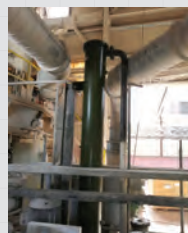
Raw Mill Gearbox
